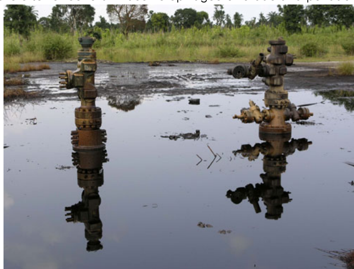
Shell’s abandoned wellheads leaking. K-dere, Ogoni. (FOEI 2006)
